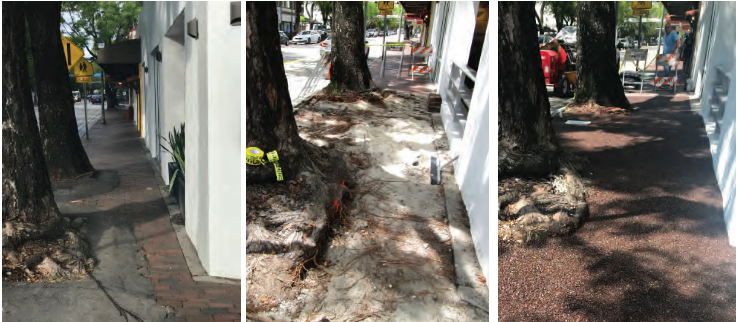
Main Highway in Coconut Grove. Sidewalks were hazardous and a temporary fix of asphalt was used by the County to try to make this passable - not meeting ADA requirements (Left). Bricks and concrete were removed to expose the root systems of the trees (Center). Flexi-Pave was installed and this area is now ADA accessible (Right).
